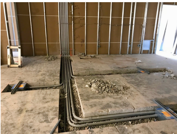
Conduits for audio wiring are being laid in the floor for Epiphany's musicians.
